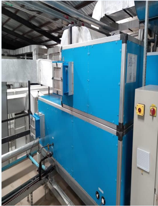
Air Handling Units, (point of dust/ antimicrobial product residue discharge at factories)
