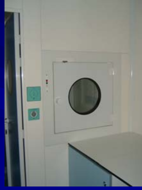
SERVICE HATCH (P3 LAB SIDE)
